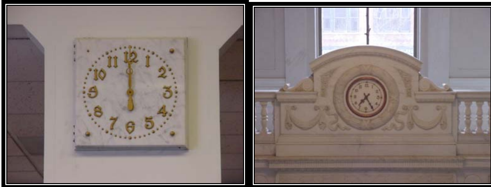
SECONDARY or SLAVE CLOCK (Division 5, Second Floor and Second Floor Vestibule)
