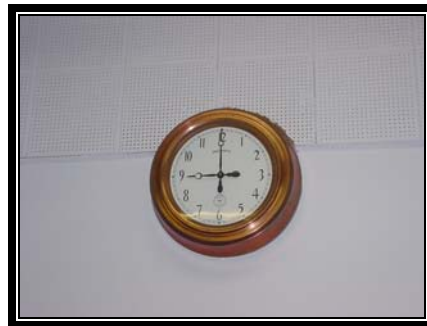
SECONDARY or SLAVE CLOCK (Administration Office, Third Floor)
